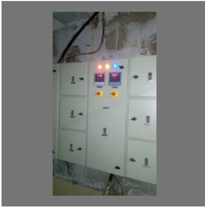
MCC Control Panel
