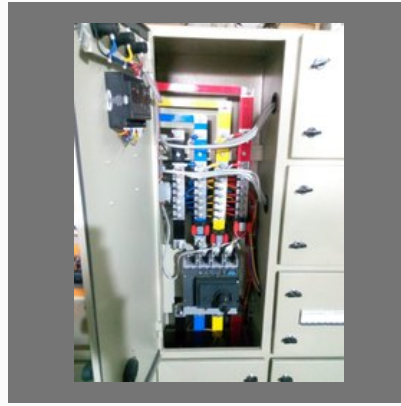
MCC Control Panel
