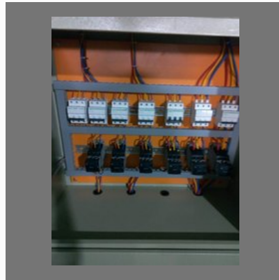
PCC Control Panel
