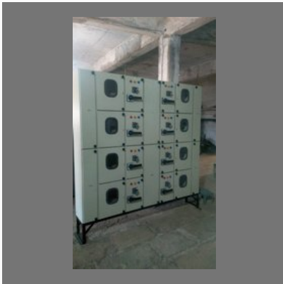
MCC Control Panel
